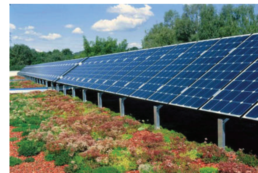
Rooftop Solar Collectors
