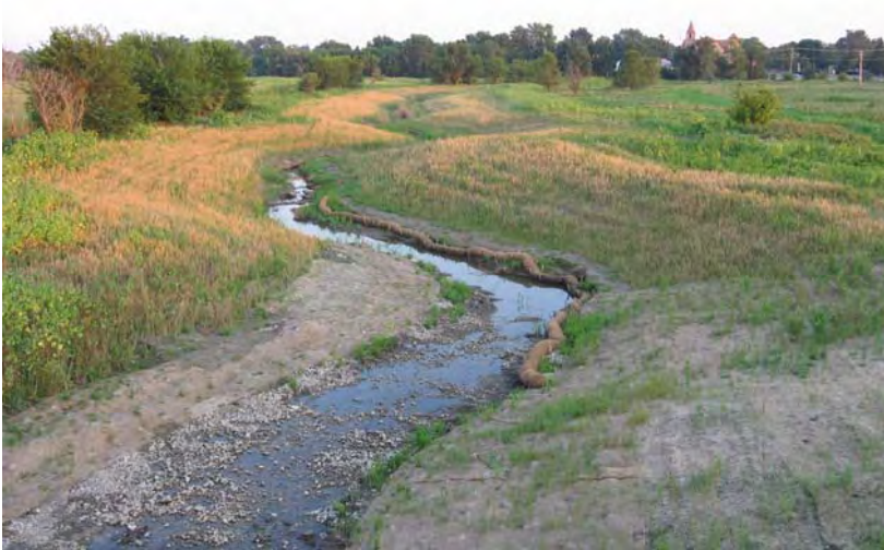
Figure 5-7. Recently completed daylighting and re-meandering project on Manhattan Creek, Village of Manhattan, Will County, August 2006.
