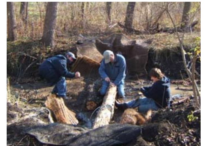
FOLA volunteers work to install a large woody debris check dam across a stream tributary to Lake Antioch (photo by R. Schieck, FOA).
