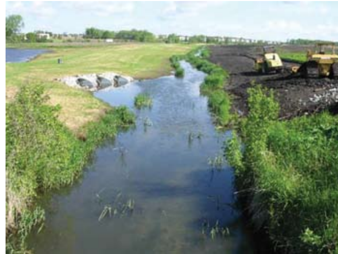
Looking upstream from Hankes Road, the re-graded banks of Lake Run are seen along with a created wetland connected to the stream in the upper left (photo courtesy of Ken Anderson, Kane County).
