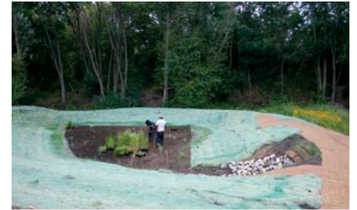
Installation of wetland plant plugs in the bottom of the constructed stormwater outfall basin (photo courtesy of Chris Tiedt, City of St. Charles).
