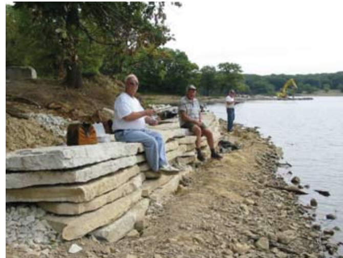
While still under construction, dedicated anglers couldn't wait to take advantage of the new flagstone protection along Maple Lake's north shore (photo by H. Hudson, CMAP).
