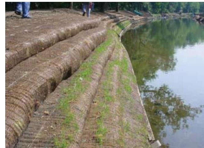
A close-up of newly installed vegetated geogrids along Salt Creek in Elk Grove Village (photo by H. Hudson, CMAP).
