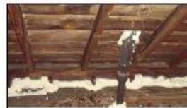
Fig. 1: Foam air sealing at rim joint and plumbing stack penetrations through attic floor
