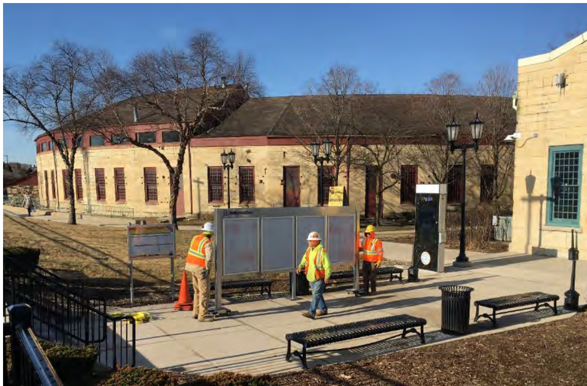
Installing the new sign structure near the historic Chicago, Burlington & Quincy roundhouse and locomotive shop
