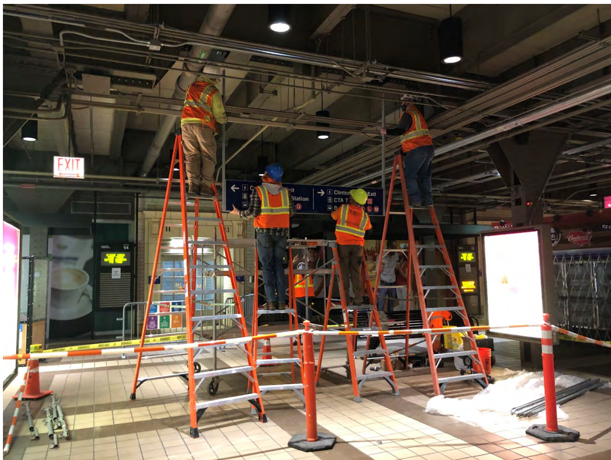
Installing a large overhead sign in the Suburban Concourse at Ogilvie Transportation Center
