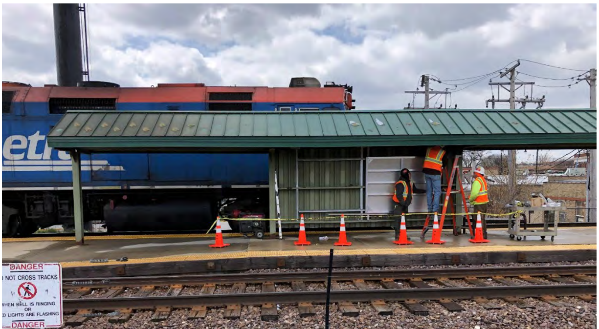
Installing the sign structure on the Metra center platform. The frame is attached to the existing wind break.
