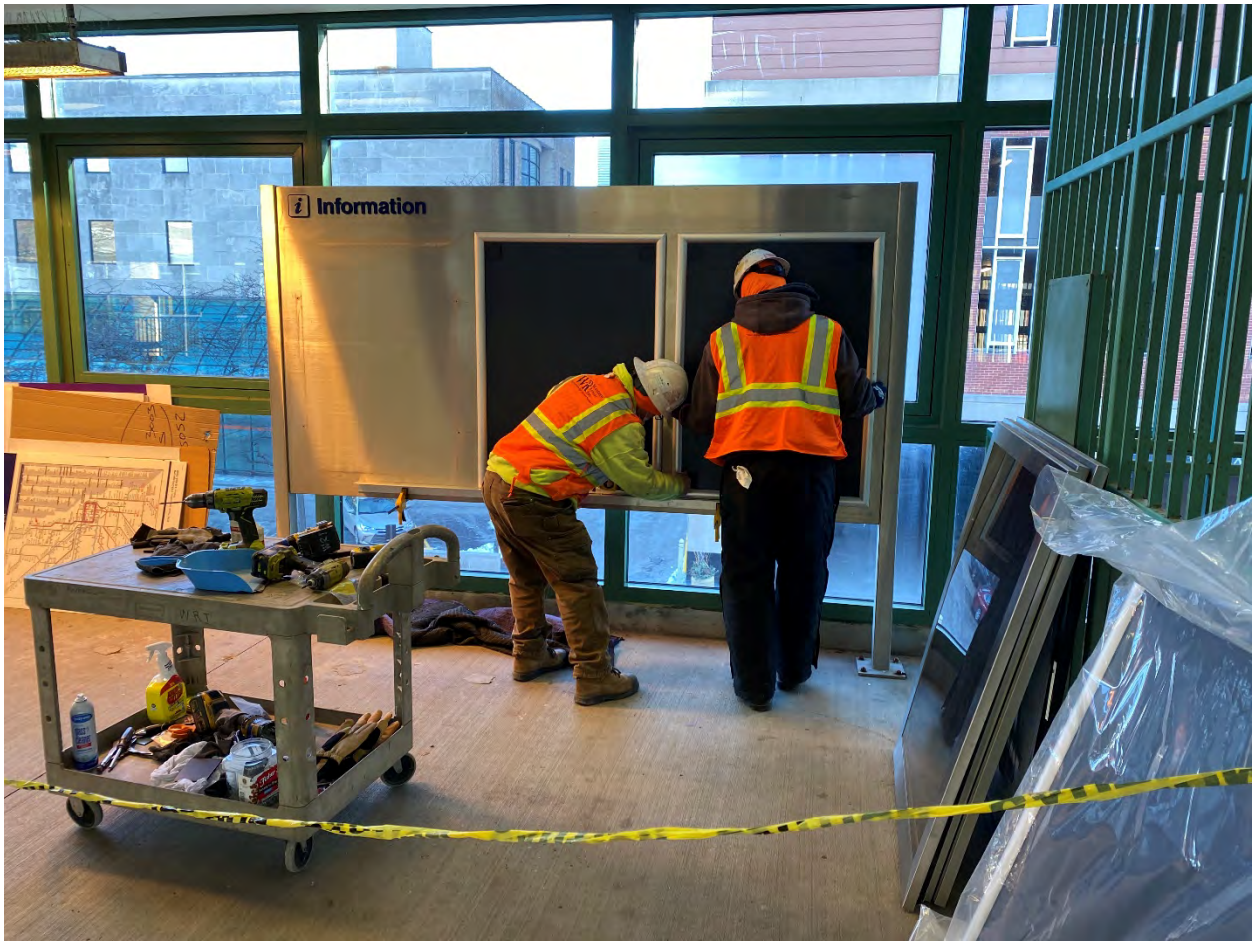
RTA maintenance contractors replacing the original stainless map frames at Davis CTA station with new aluminum snap frames.
